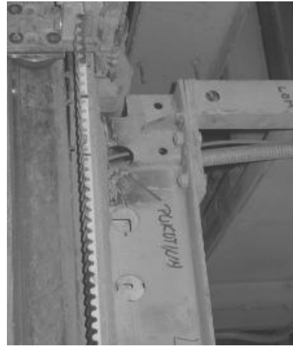
Figure 6.2: In-service crack and failure
